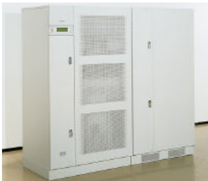
Photo 1. Powerware 9340 with battery cabinet.
